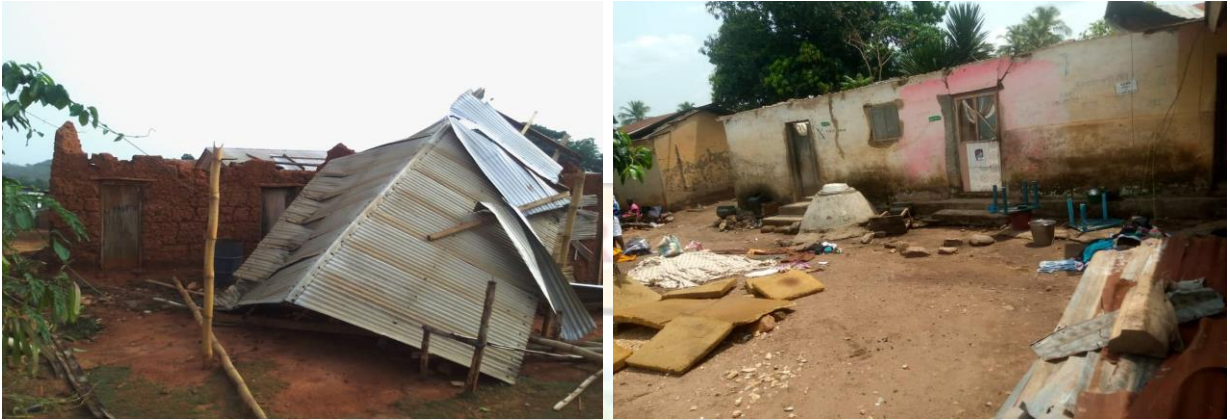
Figure 2.4.1.1 Some properties affected by rainstorm
